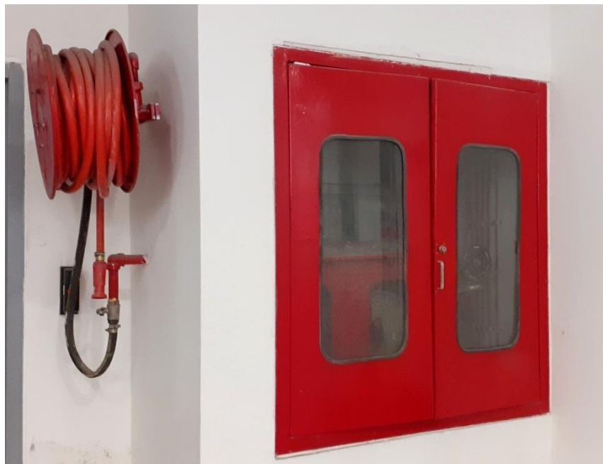
Fire Safety Equipment
